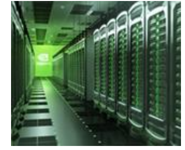
Intro to AI in the Data Center
